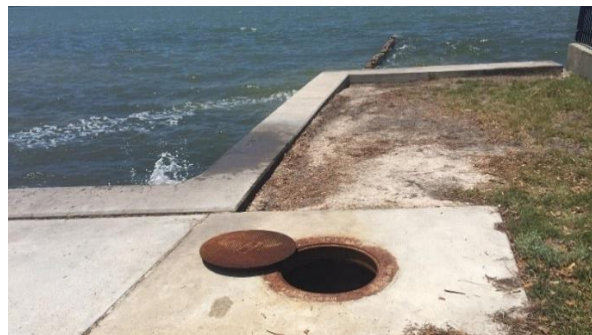
Photograph 10-3 Inline Backflow Preventors Typically Installed in the Last Manhole Before Outfall
